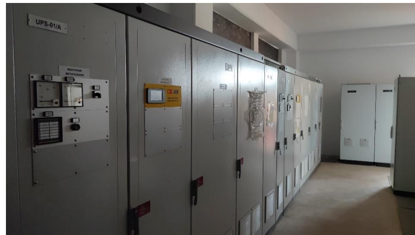
▲ AC UPS on site
