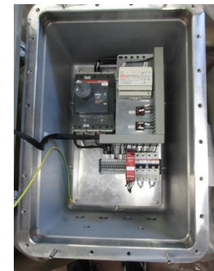
ATEX battery fuse box
