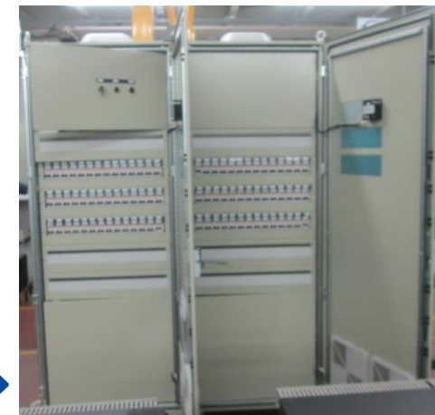
Customized DCDB (2 units) provided with n.42 MCBs
